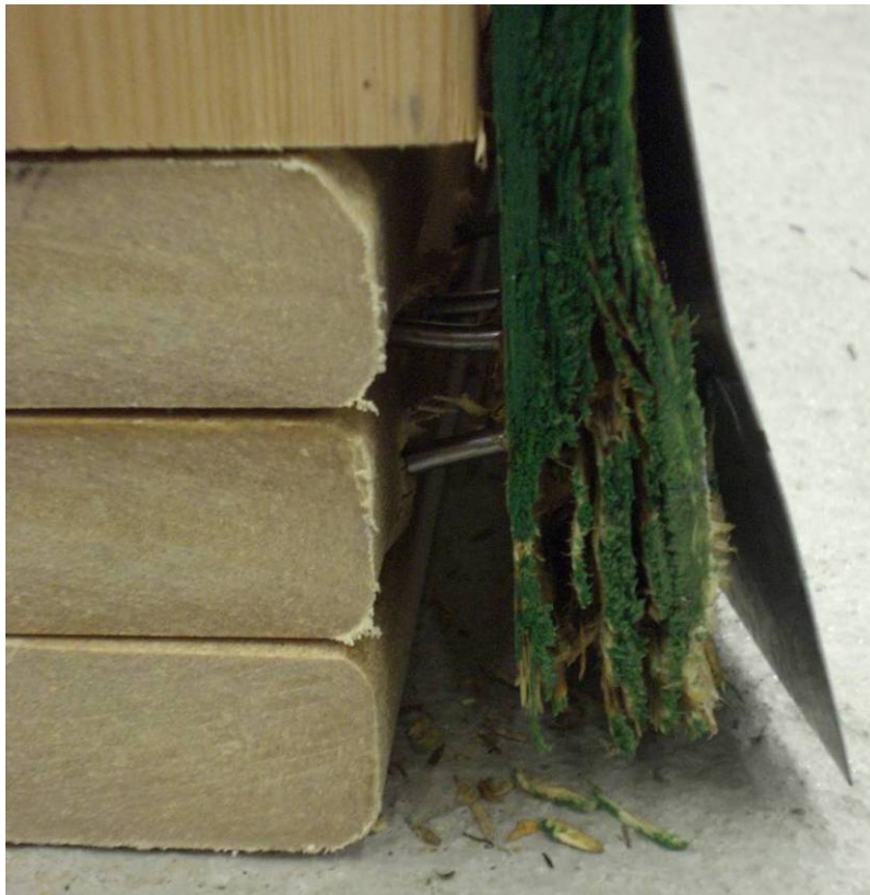
Figure 3.8 Separation of the sill plate along the melt bond
