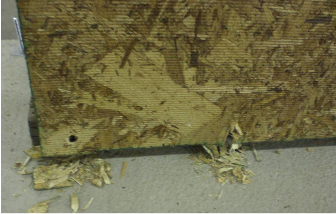
Figure 3.5 Nail head pull-through from sheathing of walls without holdowns
