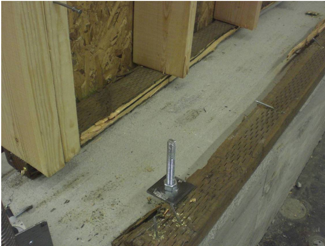
Figure 3.4 Splitting of PPT Hem-fir sill plate without holdowns
