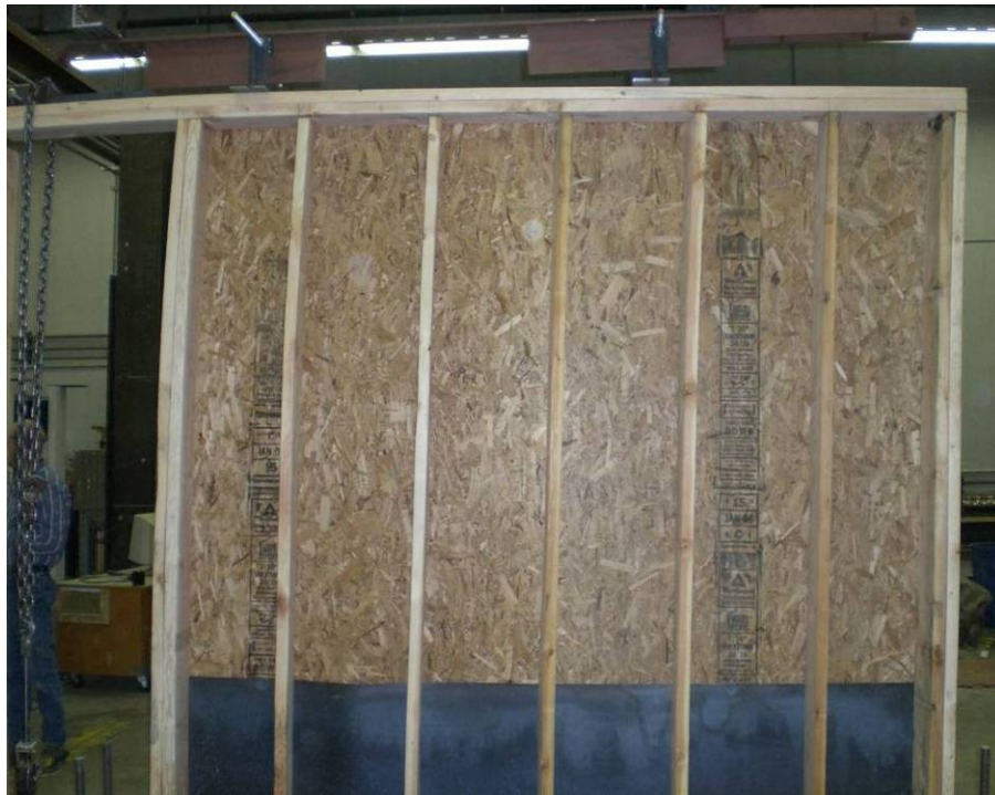
Figure 3.10 Restraint of uplift forces on the monotonic wall with a continuously embedded sill plate
