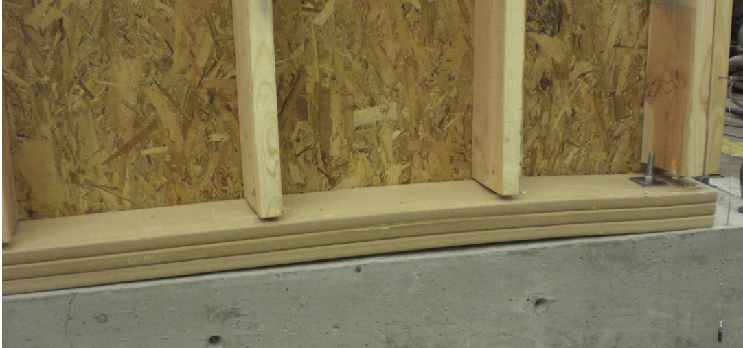
Figure 3.7 Bending of thickened WPC sill plate with triangular gusset plates (attached to other side)
